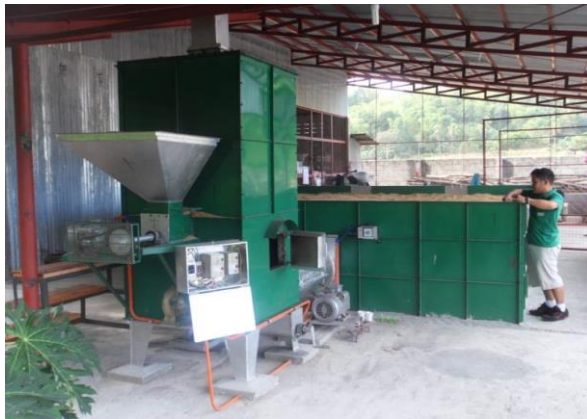
Figure 1. Installed paddy dryer on-site
