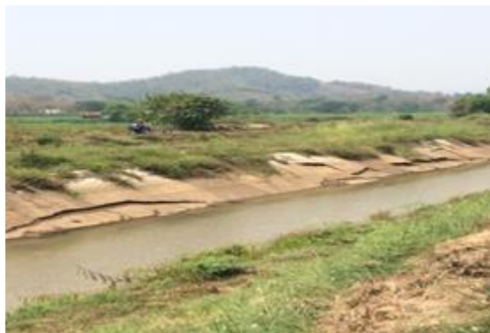
Figure 4. Broken right main canal of the Mae Lao operation and maintenance project
