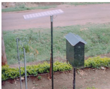
Plate 2. Energizing device (right side in box) and solar panel
